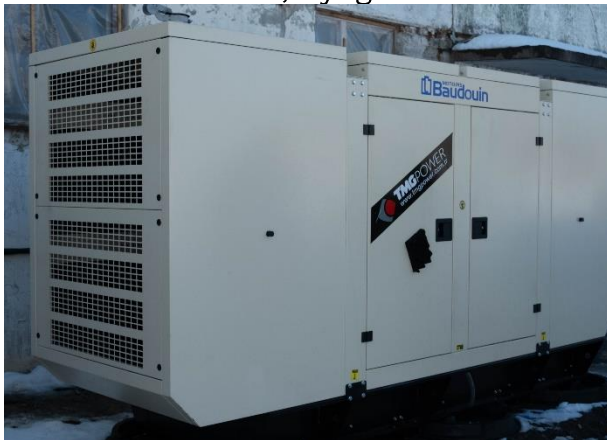
Krolevets Water supply utility - Generator 150 kW
