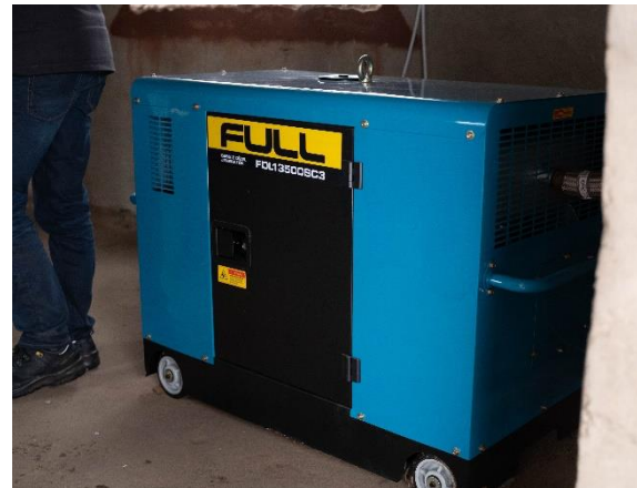
Krolevets Vocational school boiler house - Generator 11 kW
