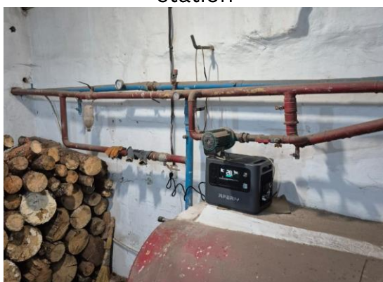
Krolevets Akvatermo (communal site) – Charging station
