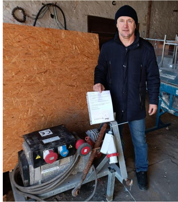
Kherson region, Municipal Enterprise “Arkhanhelske” – Generator 22 kW
