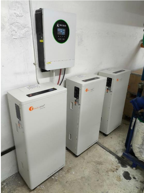
Mykolaiv city, Boiler house room - Inverter & batteries
